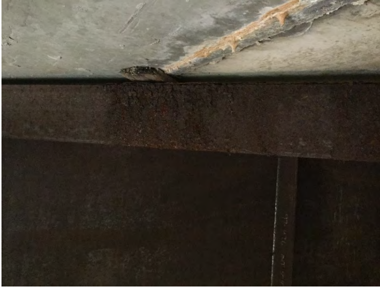
Minor bracing corrosion
